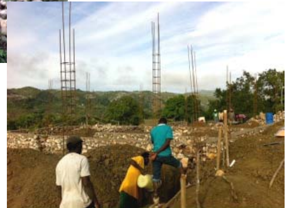
Below: St. Rose of Lima foundation and structure.
